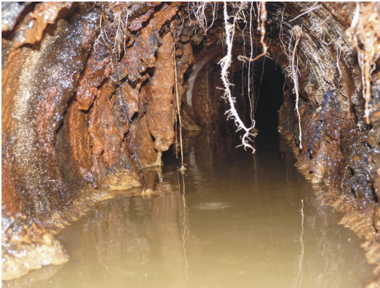
Fig. 4. Ferruginous substance in a pipe
